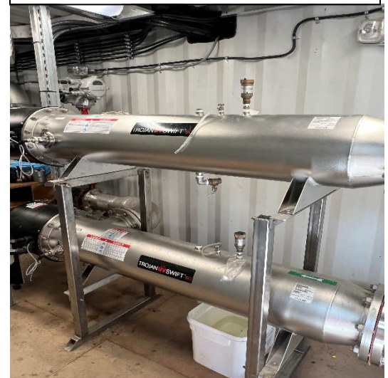
Trojan Swift UV Reactors
