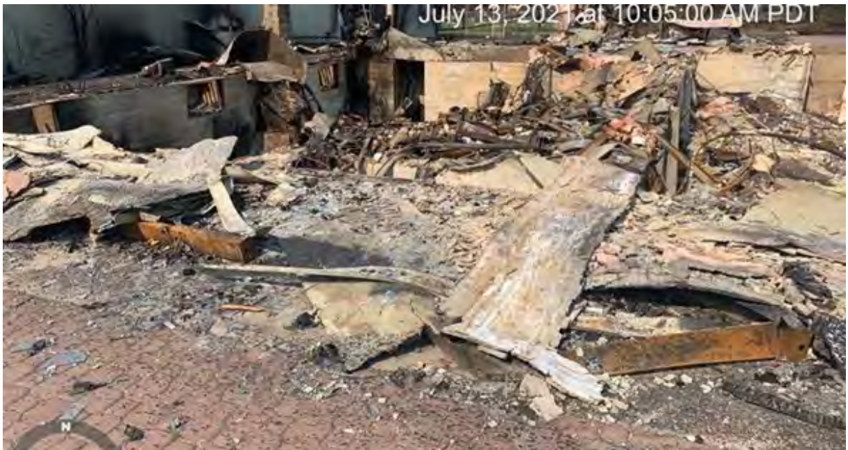
Photo 3 View of suspected asbestos | Facing west | July 13, 2021
