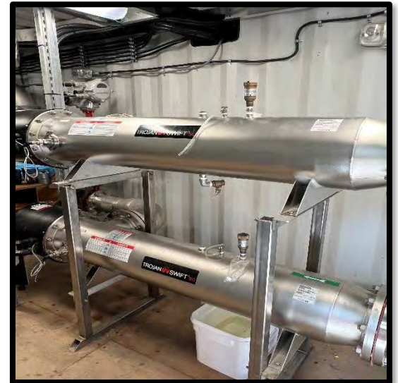
Trojan Swift UV Reactors
